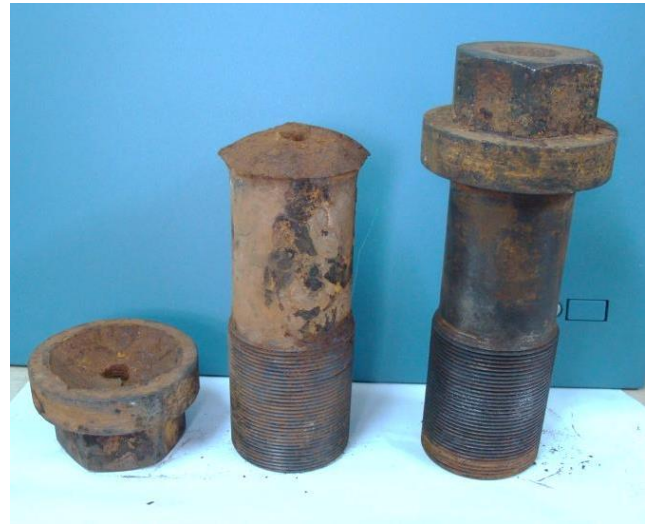
Fig. 1 – Bolts for mounting the runner of the turbine (M110x4) after 30 years of operation
